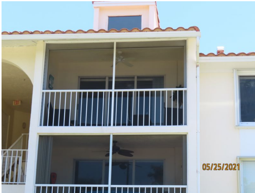
Unprotected Glazed Entry Door
