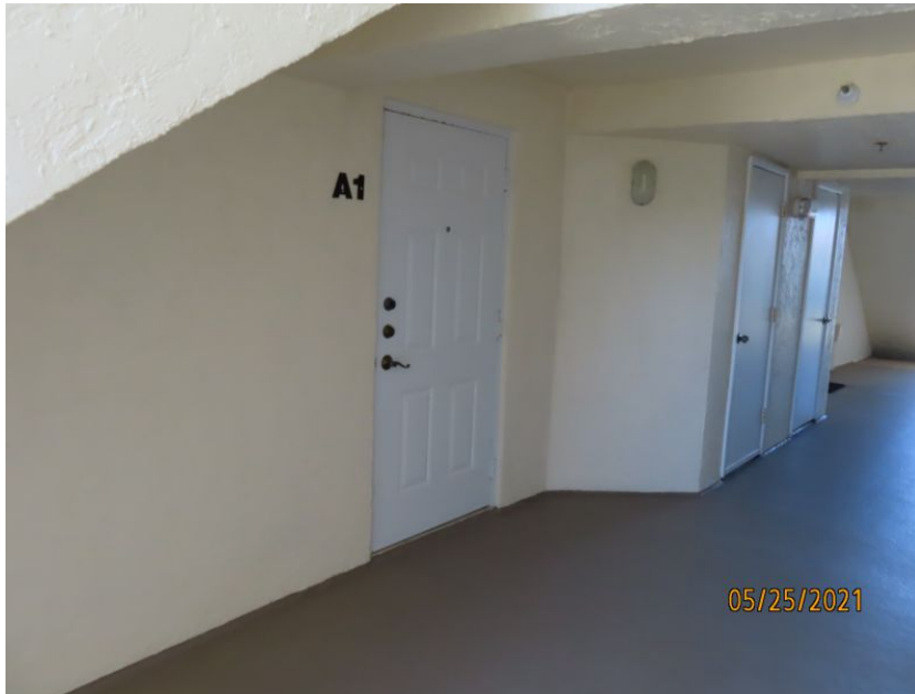
Unprotected Solid Entry Door
