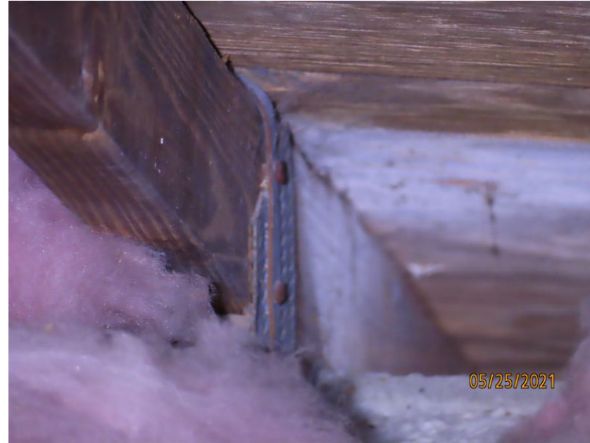
Metal Connector with 3 Nails on the Front Side & 0 Nails on the Opposing Side
