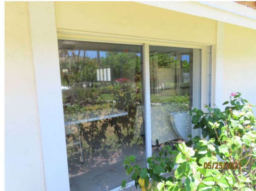
Unprotected Glazed Entry Door
