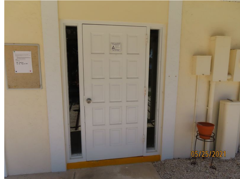
Unprotected Solid Entry Door
