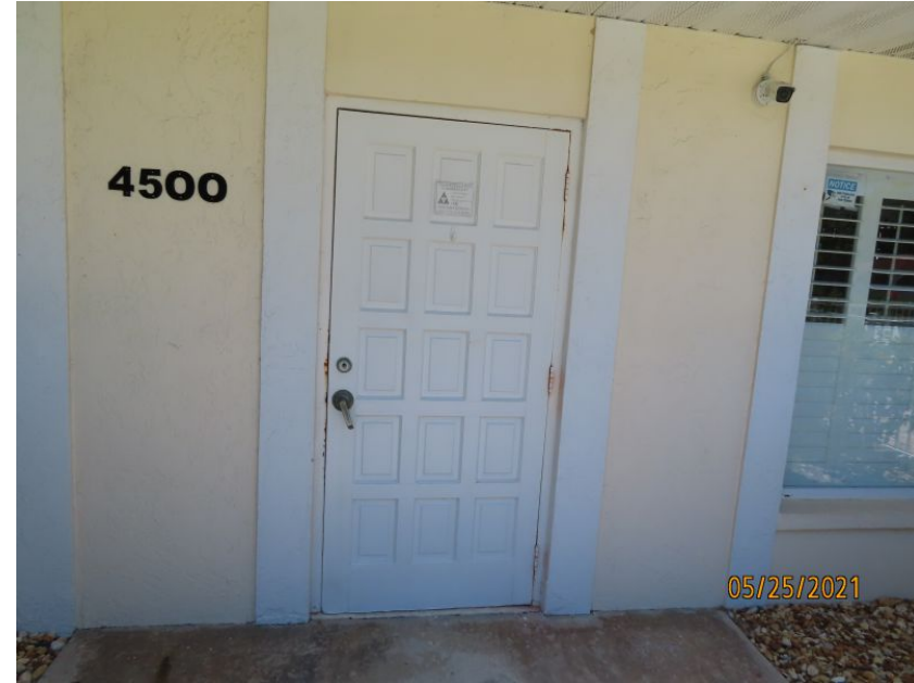
Unprotected Solid Entry Door
