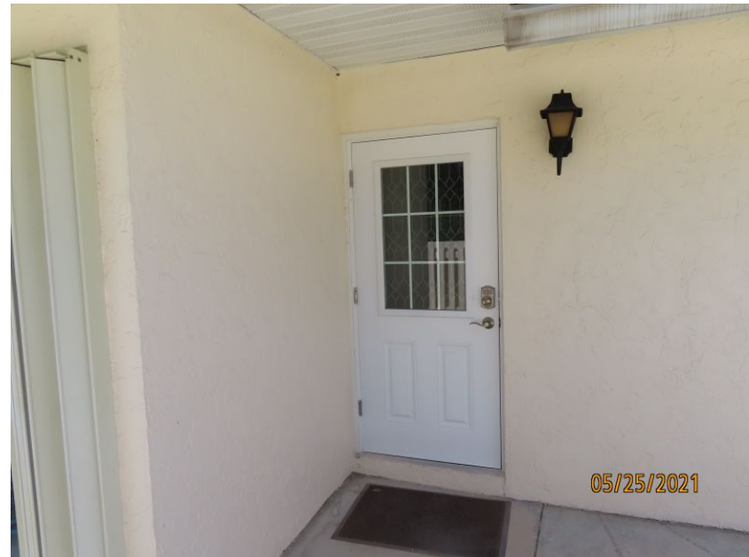
Unprotected Glazed Entry Door
