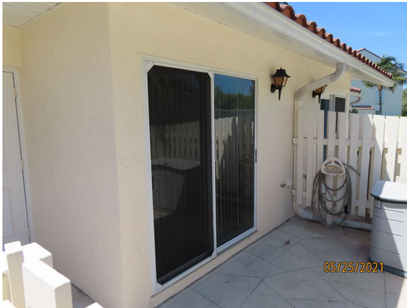
Unprotected Glazed Entry Door
