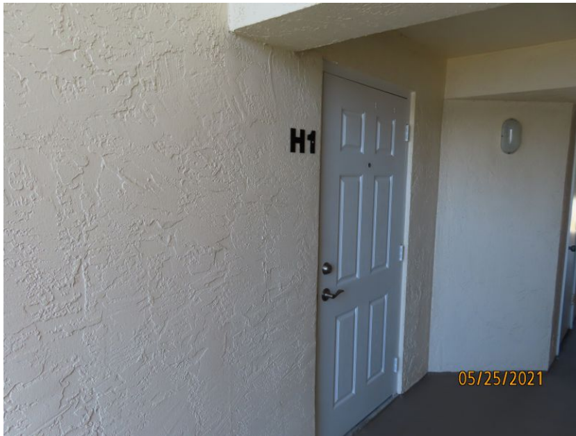
Unprotected Solid Entry Door
