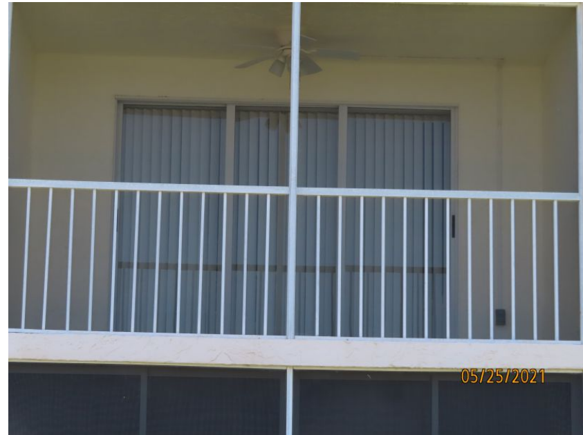
Unprotected Glazed Entry Door
