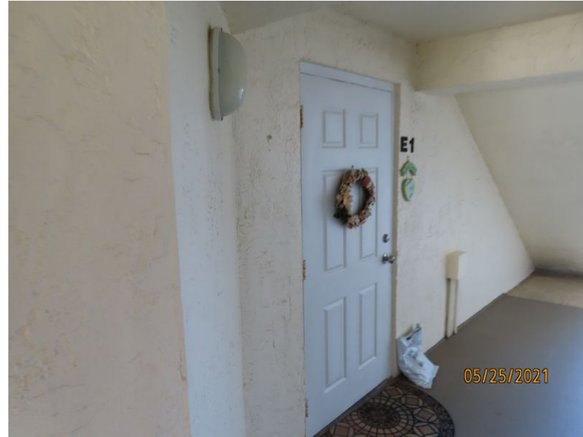
Unprotected Solid Entry Door
